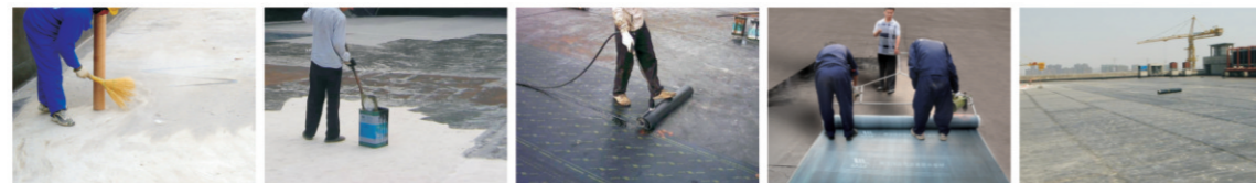
1. Treatment substrate 2. Paint substrate agent 3. Hot melting construction 4. Width membrane hot material construction 5. Complete spreading and paving
